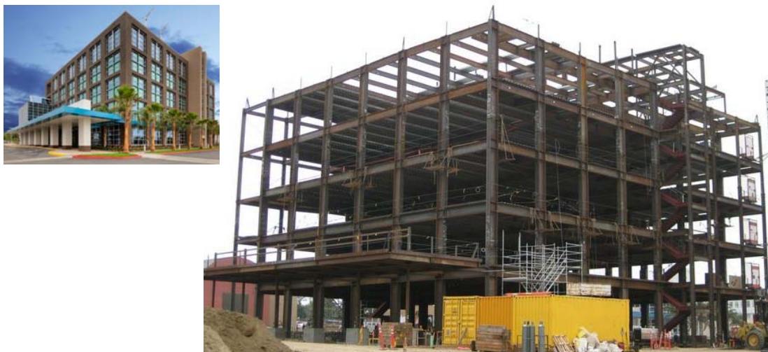
Figure 1.1: A building with steel SMF as lateral load resisting system (Ventura County Medical Centre, Ventura) [Photo credit: Wheeler and Gray, 2019]
